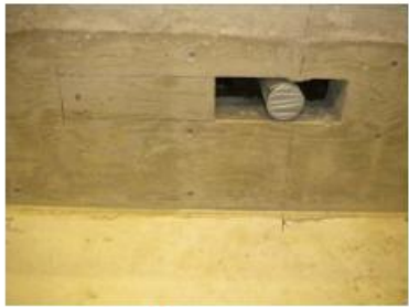
Conduit in Wrong Place
