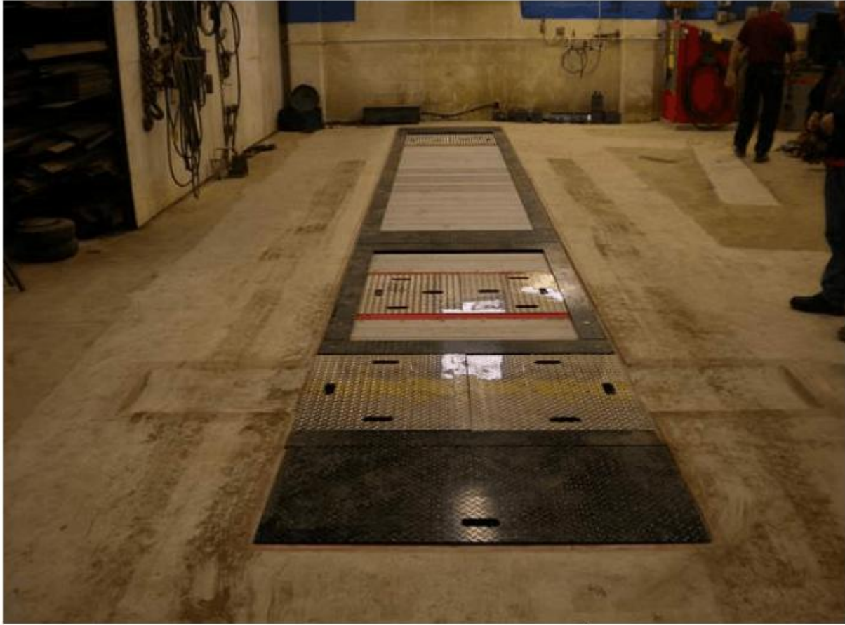
Minot DOT Installation completed Oct. 28 th , 2009
