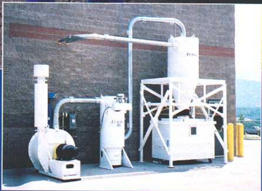
Centrifugal Eurovac multi-stage pump with multiple cartridge filters and automatic compressed air "pulse-jet" cleaning (with pre-separator depositing debris directly into dumpster).
